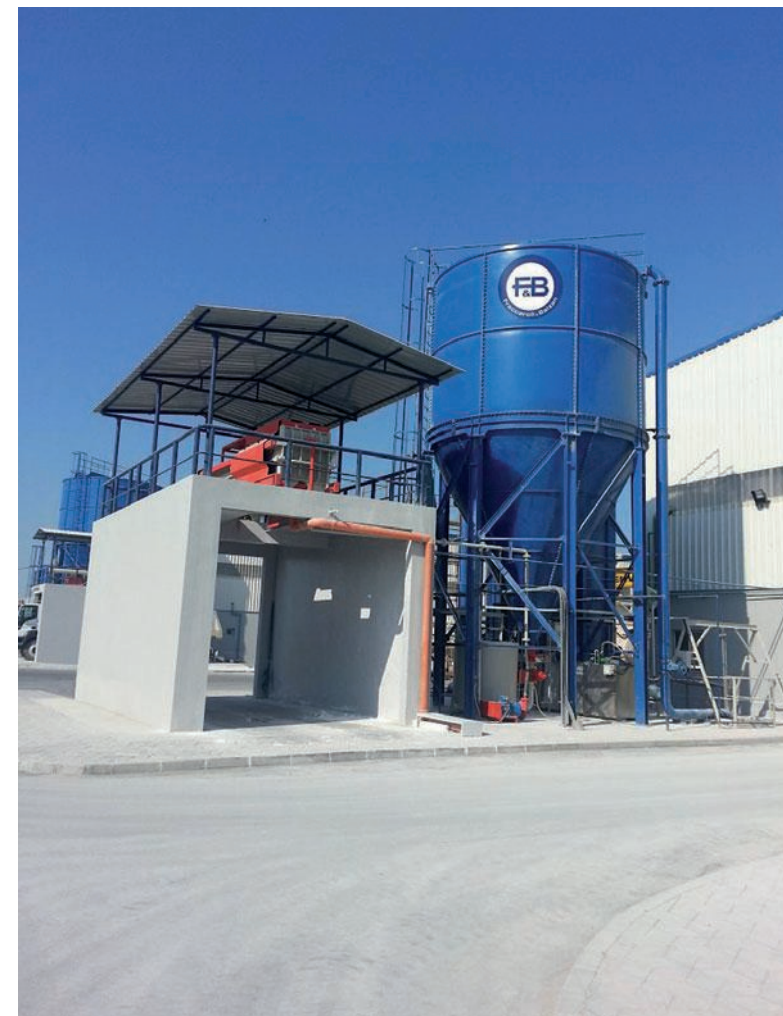
Waste water treatment plant for the TILE LINE
