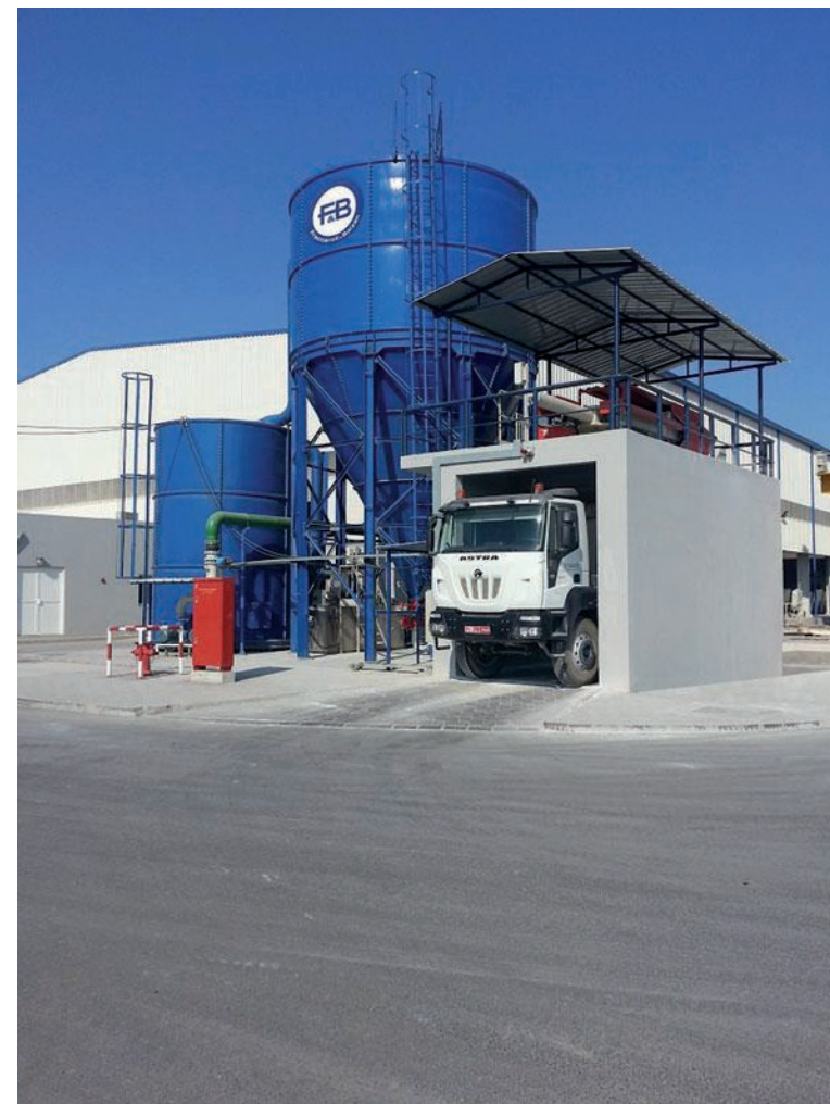
Waste water treatment plant for the SLAB LINE
